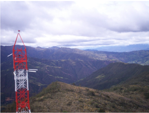
Figure 2. EBSA Repeater No. 2
