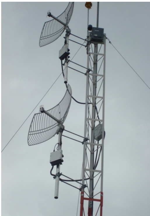
Figure 4. 195Eg Repeater Site
