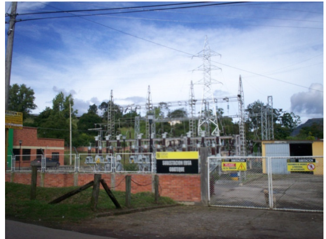
Figure 1. EBSA Primary Substation No. 1
